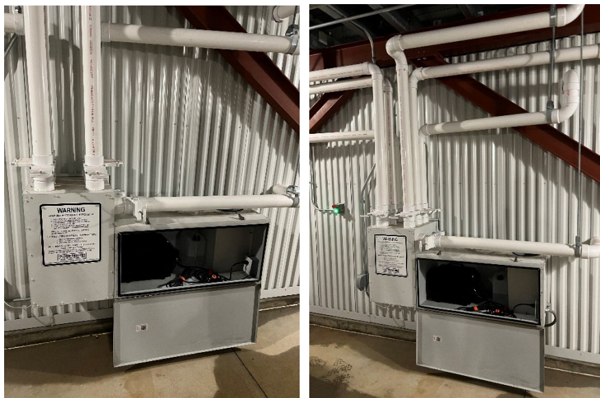
Centralized 70,000 cfm Smoke System w/ Blower and PVC Distribution
