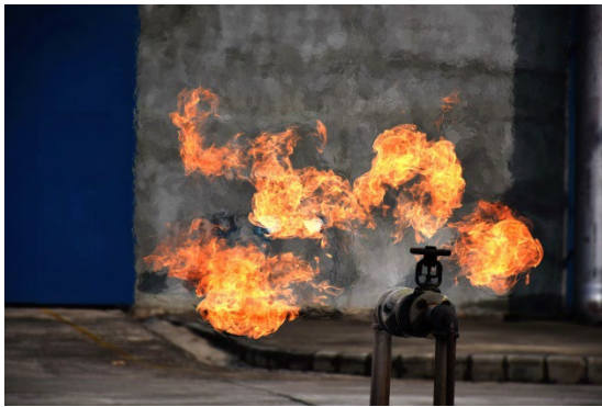
ST Split Flange Fire
